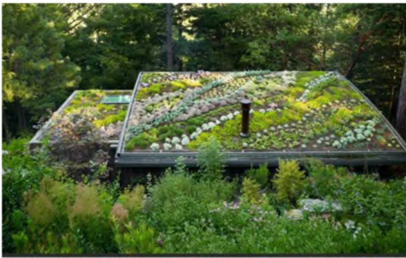
Vegetated roof slows stormwater runoff.
