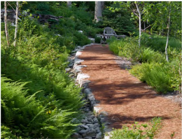
Infiltration trench paralleling a pathway.
